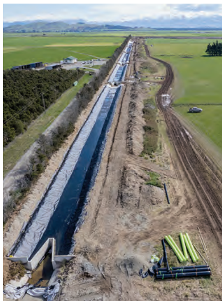
Lining a significant section of the primary water race at Te Whenua Hou.
