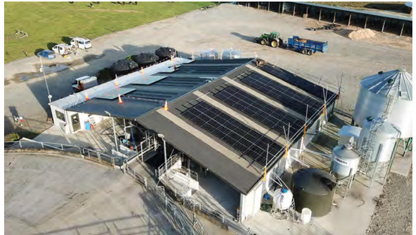
Solar Installation at Hamua Dairy Shed, Te Whenua Hou Te Whenua Whitiorea.
